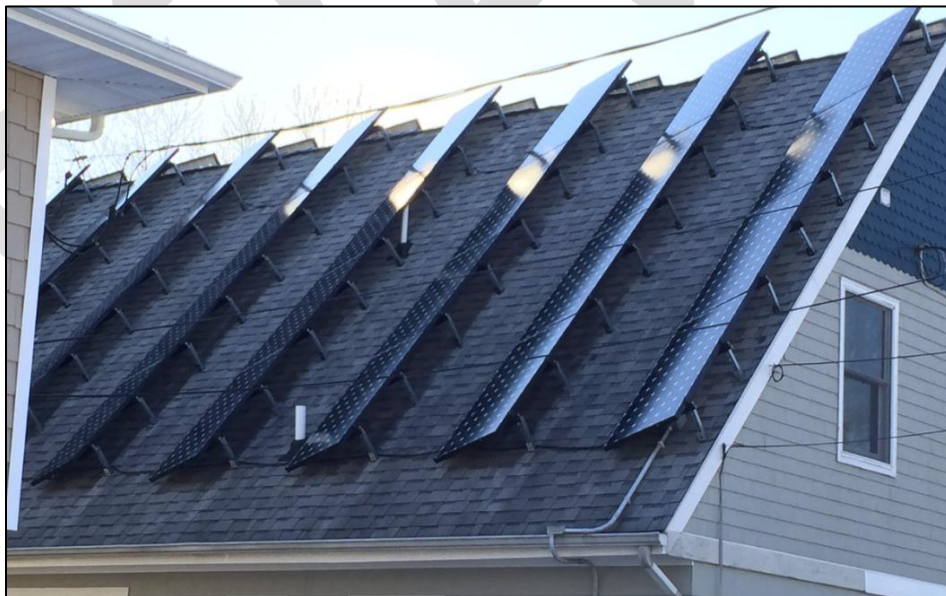
Panels not mounted parallel to the slope of the roof and not flush with the roof.
